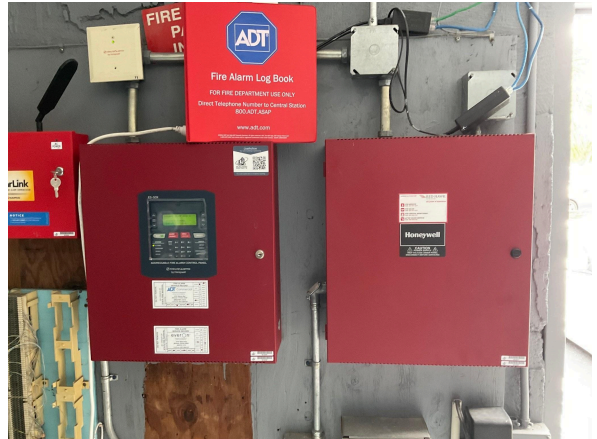
Fire suppression equipment
