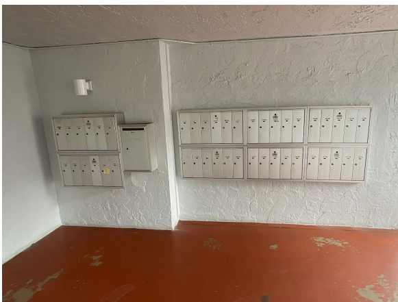
Mailbox kiosks and common area lighting
