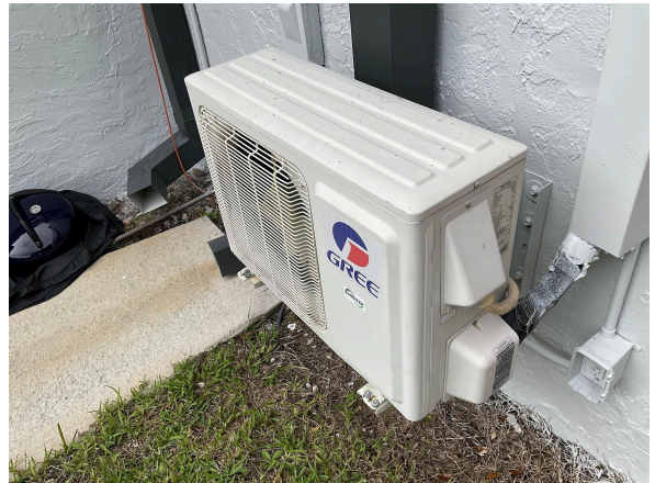
Common area HVAC equipment
