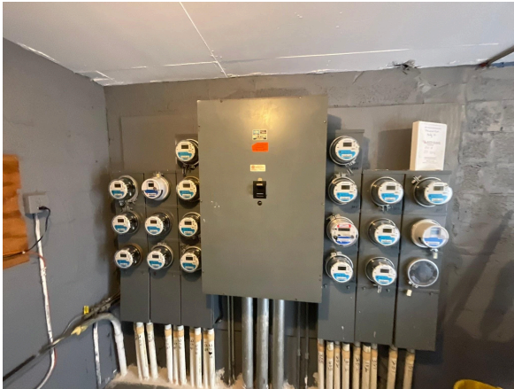
Electrical equipment room
