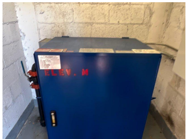
Hydraulic elevator pump
