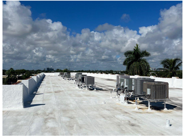
Rolled modified bitumen roof
